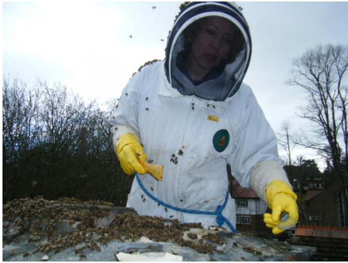
The chimney had a slate capping but bees had found ways in through cracks in the cement.
